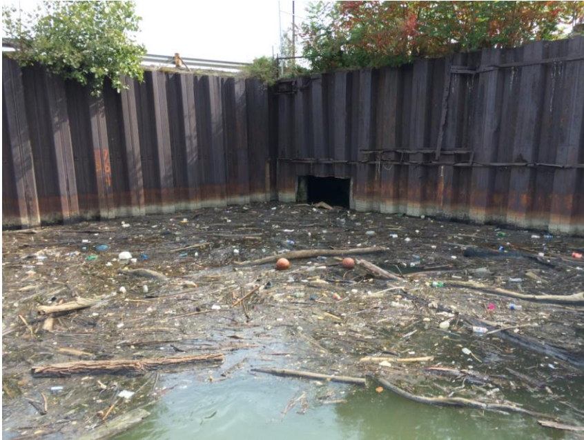
Visible storm debris at Combined Sewer Outfalls (CSOs) in the Ship Channel
