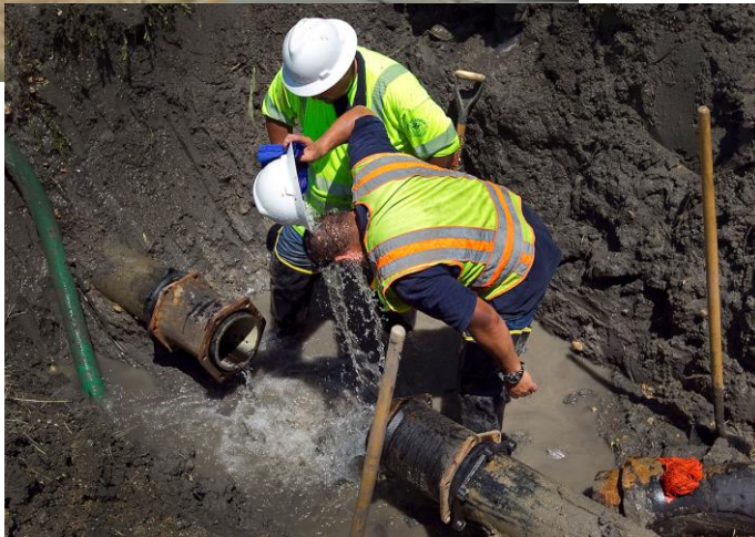
Bastrop County Fires and Burst Pipes.
